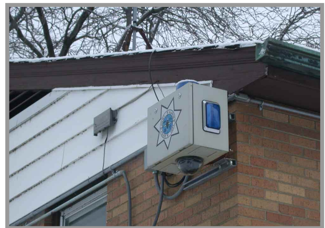
ARVIS with Toshiba IK-DP30A dome camera installed at townhouse project (Joliet, Illinois)
